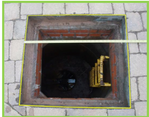
*Incorrect installation and measuring of a clear opening
